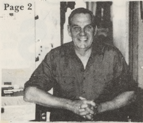
Kenny Hendrickson at his desk in the boiler room at North Shore Elementary.
